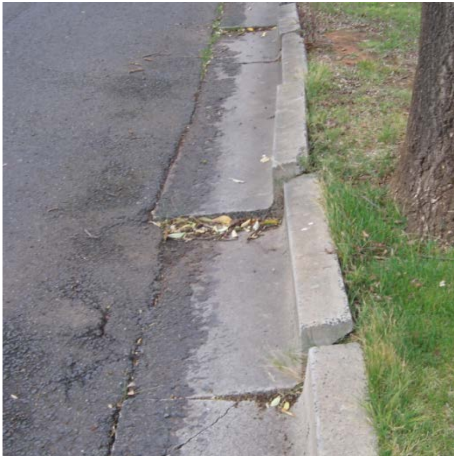
Figure 21: Legacy of past construction practices
