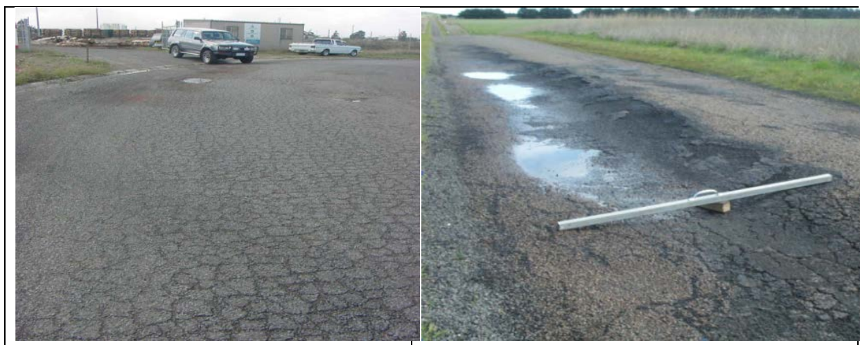
Figure 10: Examples of severe ( ) & significant ( 3) Cracking and Rutting
