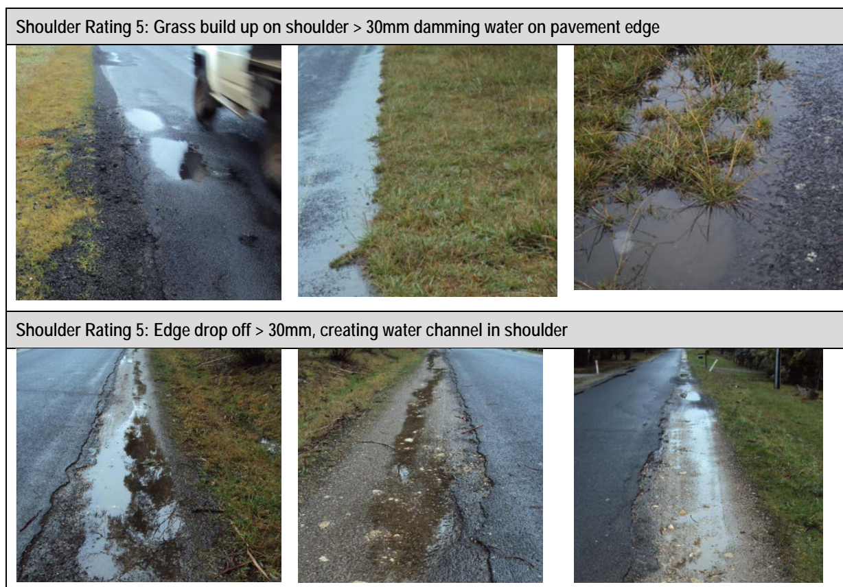
Figure 11: Examples of Shoulder Condition 'Failed'
