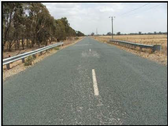
Condition 6.5 - 7 Oxidized and Stripping
