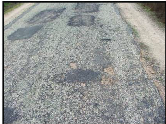
Condition 8 Fully Oxidized and falling apart
