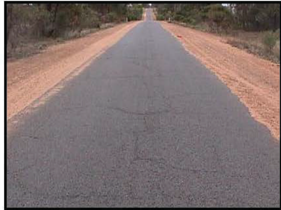
Condition 5 Cracking but seal not too oxidized
