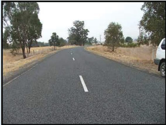
Condition 0 – 1 Seal in Excellent near new condition
