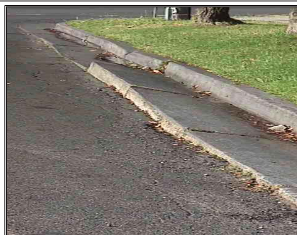
Condition 9 Extreme movement and lack of Function
