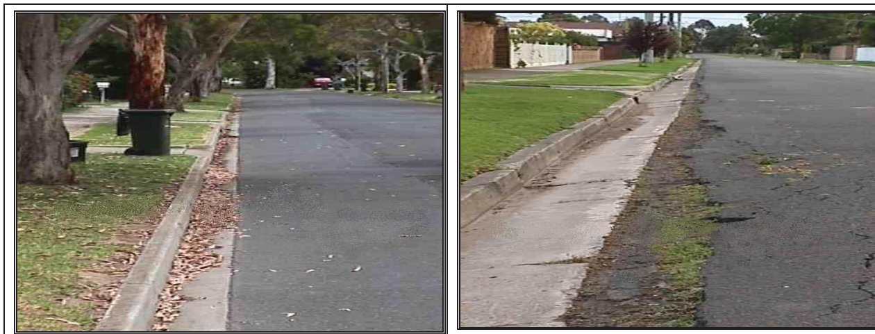
Condition 3 Old But only Minor loss of shape & movement
