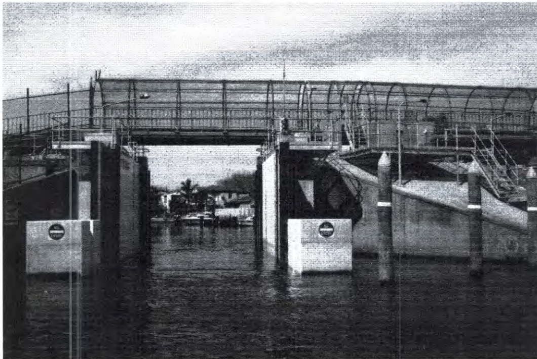
Figure 14: Tidal floodgate to the Tidal Waterways looking from the Patterson River into Whalers Cove.
